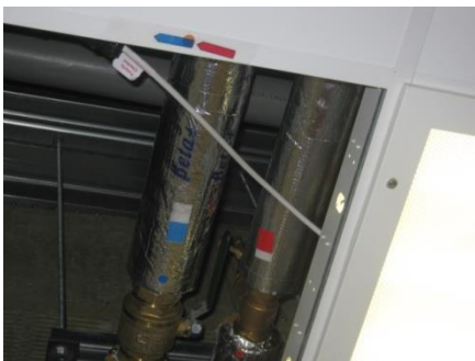
Valves above ceiling next to main door
