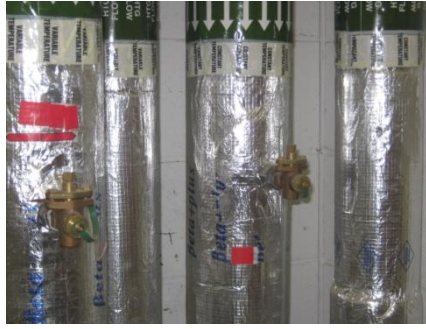
Hot water valves (Left hand side main)
