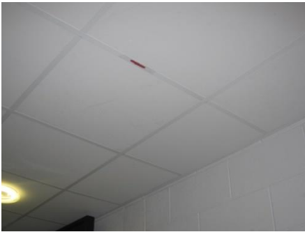
Ceiling marking which is near TV screen in restaurant
