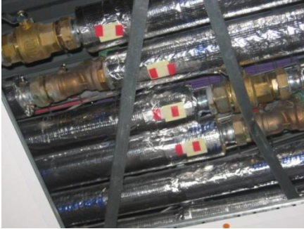
Valves above ceiling
