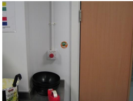
Gas shut off valve – Kitchen behind main door
