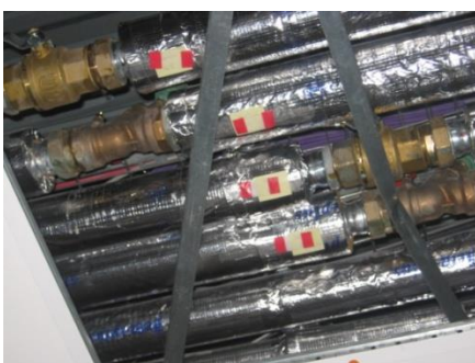
Hot water isolation valves
