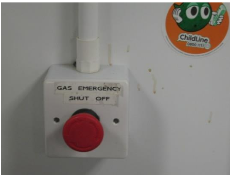
(Gas shut off valve – Kitchen)
